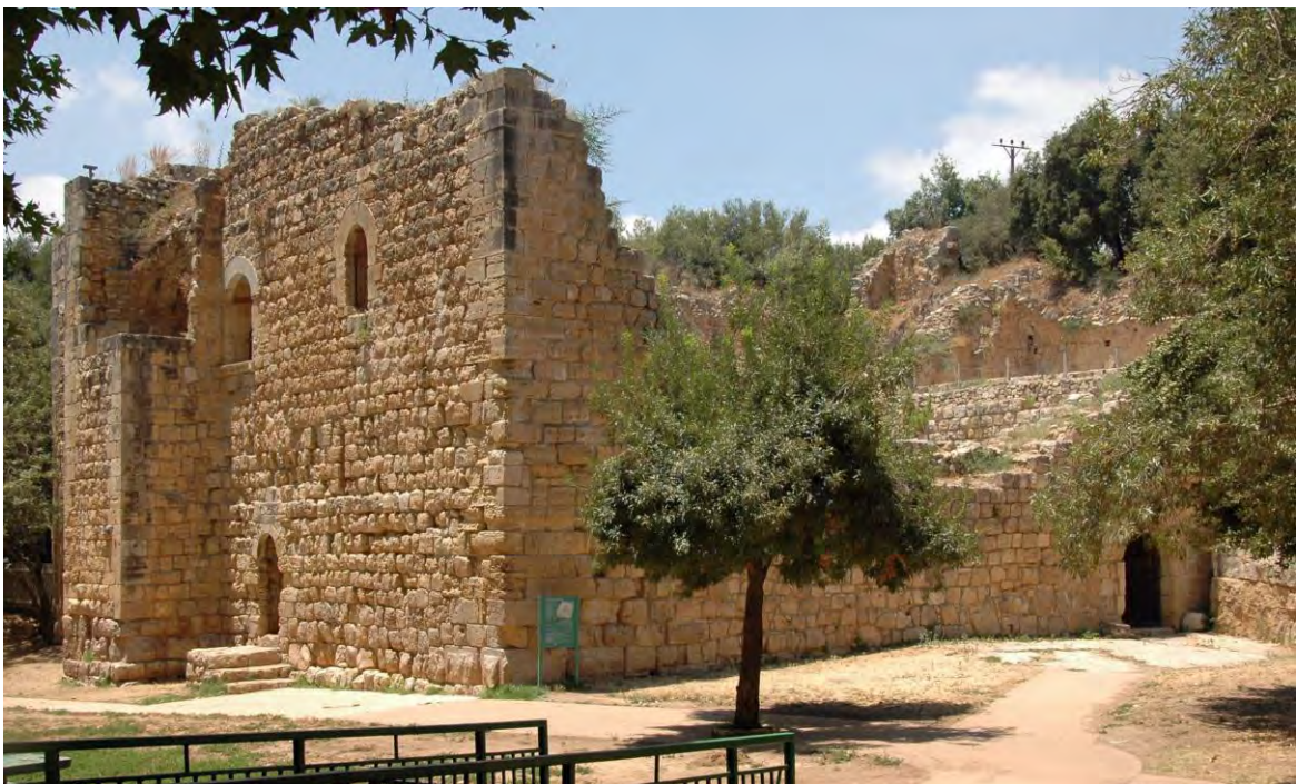
Fig. 4 – Aqua Bella (Kh. 'Iqbalā): a Frankish manor house, converted into a monastic infirmary by the Hospitallers after c.1140 (© DP 2013).
